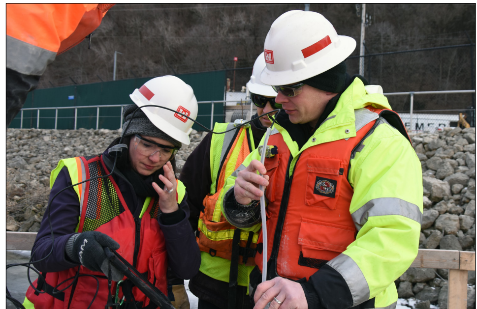
(Left to right) Project manager Kim Warshaw and engineers Jake Fall and Wade Carr, use a remote camera to inspect a void in the upstream guidewall at Lock and Dam 8 near Genoa, Wisconsin, Jan. 8.
